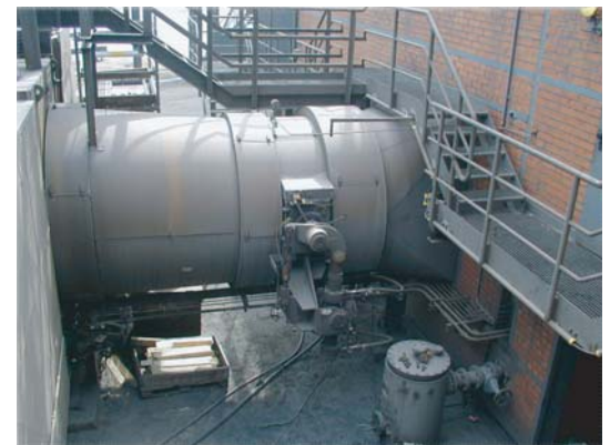
Main Stop Valve
