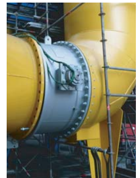
Main Stop Valve (detail)
